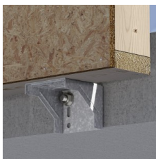
Bracket below, in the middle of concrete
